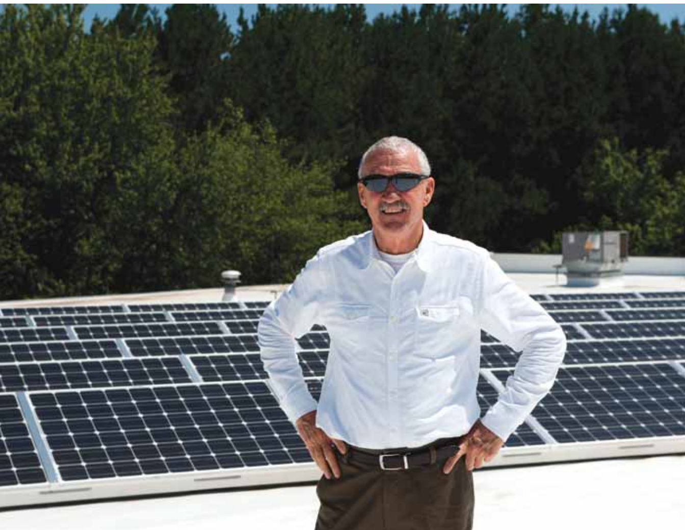
As part of the Georgia Non-Profit Solar Project, Radiance Solar installed 105 solar panels on our Southeast Region Distribution Center.
